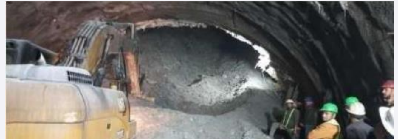
Silkyara Tunnel after the collapse
